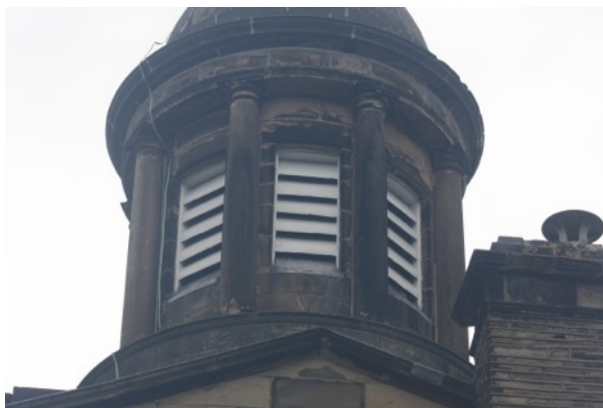
View of the Bell Tower from the South - grey mesh visible at the bottom of the louvres Aug 2021
