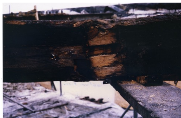
Original fractured timber bottom chord after removal of straps and bolts
